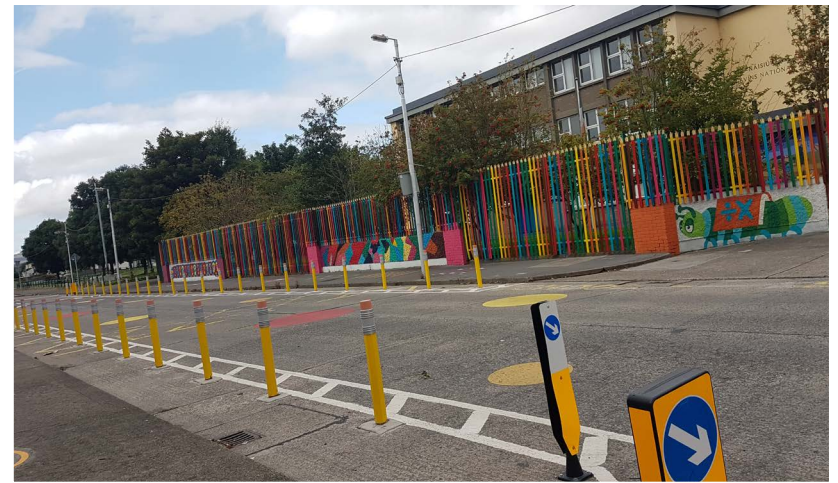
In consultation with local children, we transformed the school railings of St. Kevin’s and St. Joseph’s Schools, Finglas into colouring pencils, painted murals designed by the children and play markings on the footpaths leading to both schools
